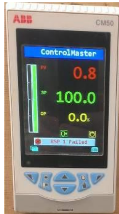
New PID controller
